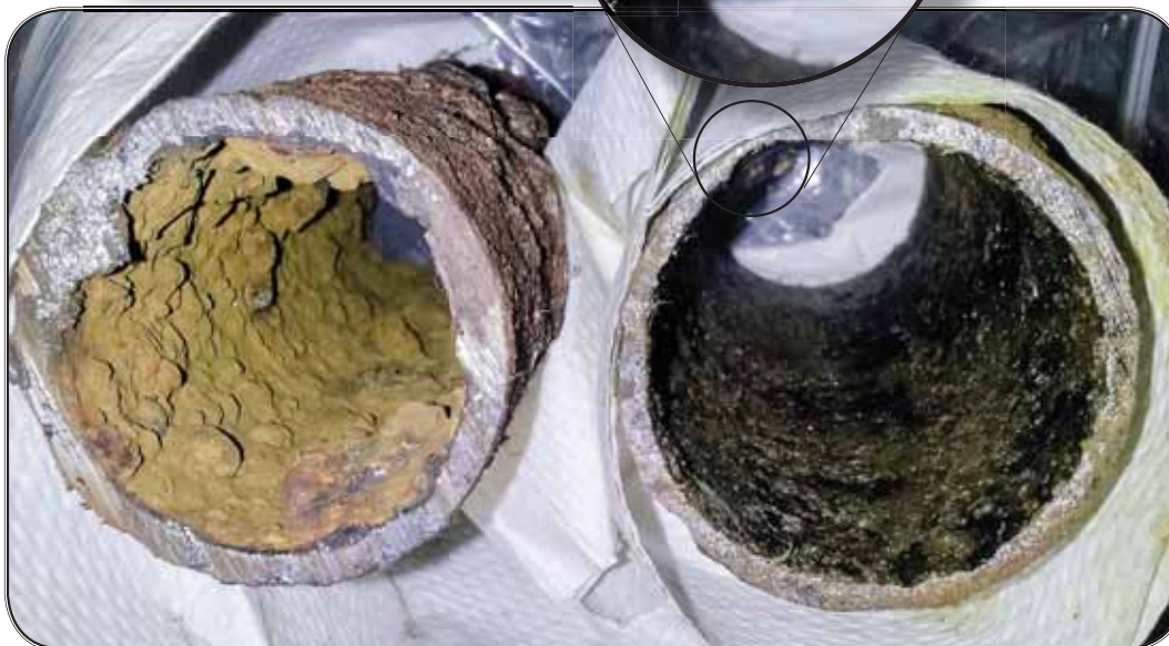
Under-deposit corrosion thins pipe walls
